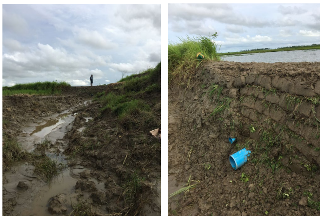
Figure 12 Rebuilding of expensive man-made barrier after heavy water flooding in a non-beneficiary farmer's field at Boyargyi village (September 2018)
